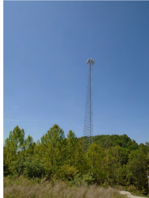
Photo 30: Cell tower engine on northern portion of property. Orientation: North facing view
