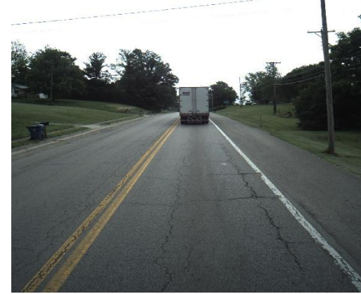
Longitudinal Cracking = Poor
