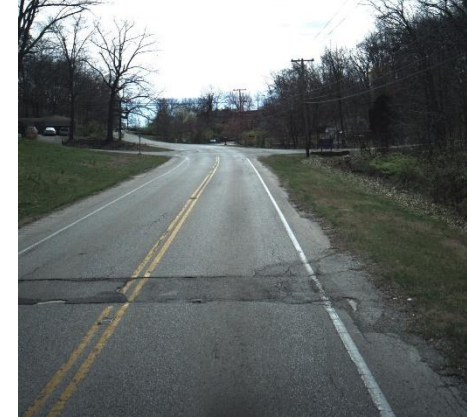
UTILITY CUTS = POOR
