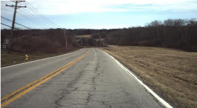
PATTERN CRACKING = POOR
