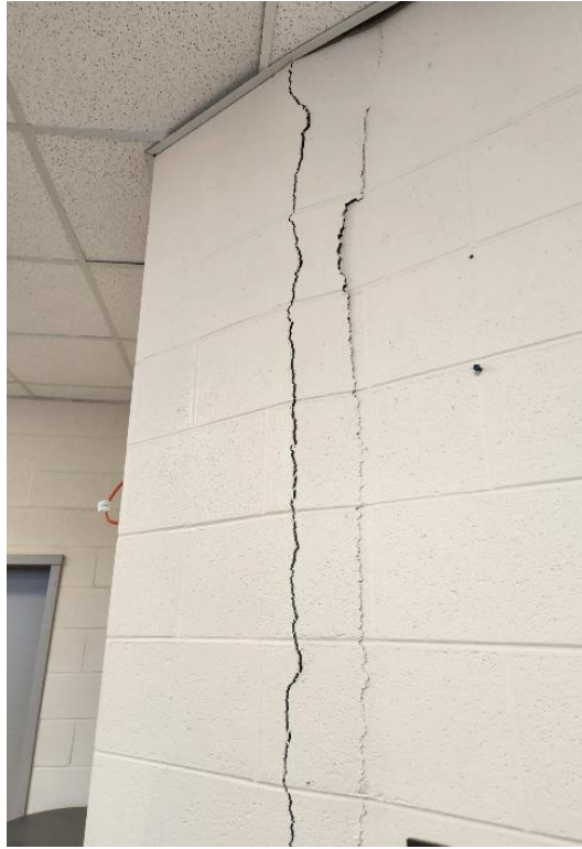
Photograph 7: Upper-level cracking in front room.
